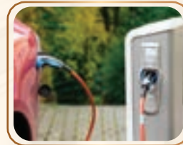
Electric Vehicle Charging Point
